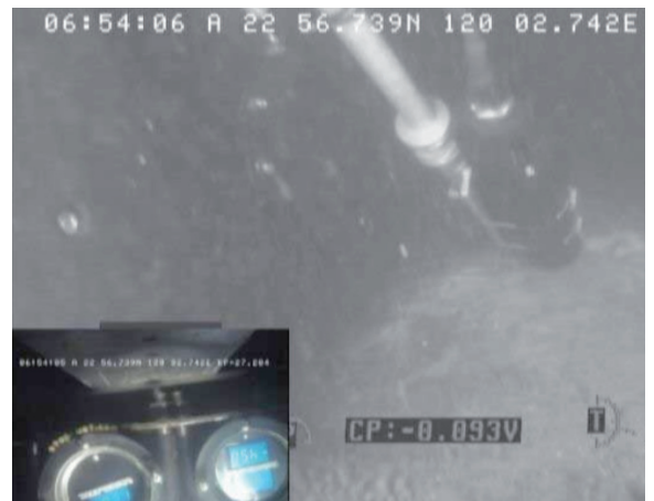
Subsea photo Taken during a CP survey using dual Deep C Meter readouts
